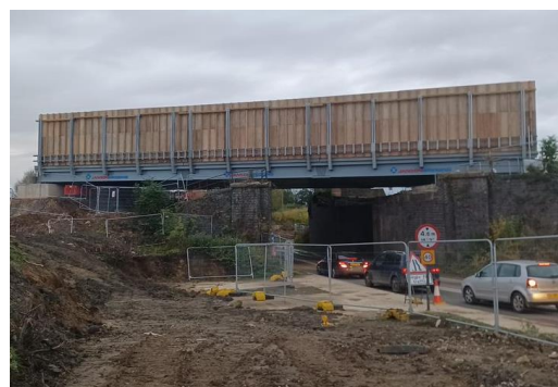
Example showing the temporary bailey bridge that was constructed for our construction vehicles to cross the A4421.
